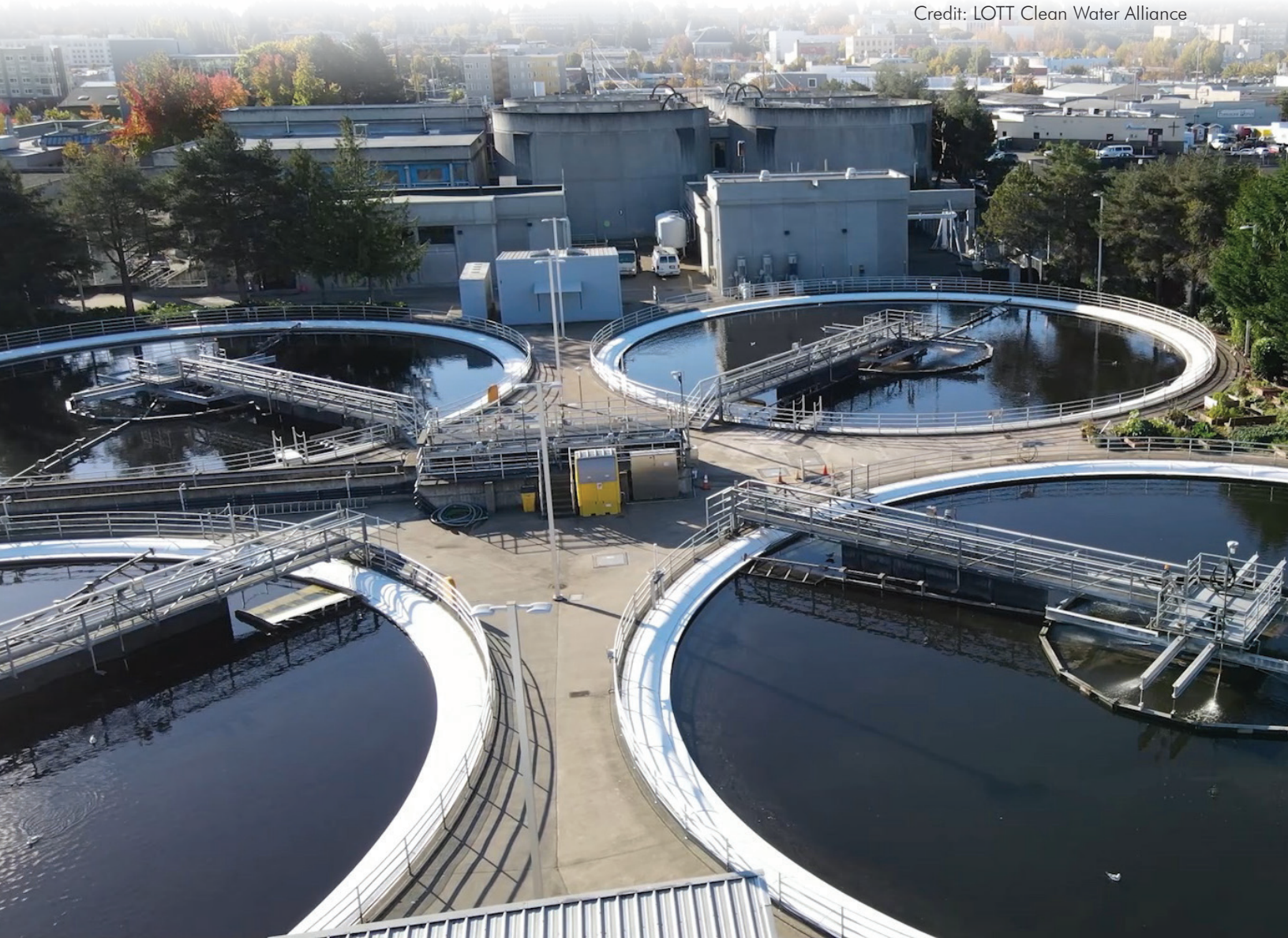
Secondary Clarifiers and digesters at the Budd Inlet Treatment Plant. Credit: LOTT Clean Water Alliance
